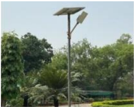
solar lights installed
